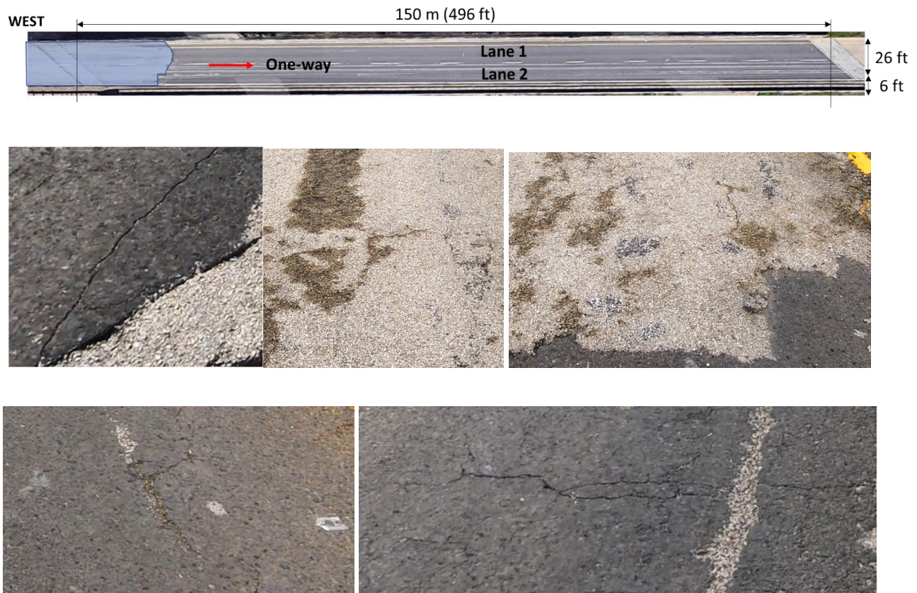
Figure 6.17. Bridge scanning and surface defects visualization: The 3DGPR system covers a 150-meter length and 4-meter width area, employing four scanning paths (Lane 1 and Lane 2). The bridge deck exhibits multiple surface damages, including cracks and spalling.
