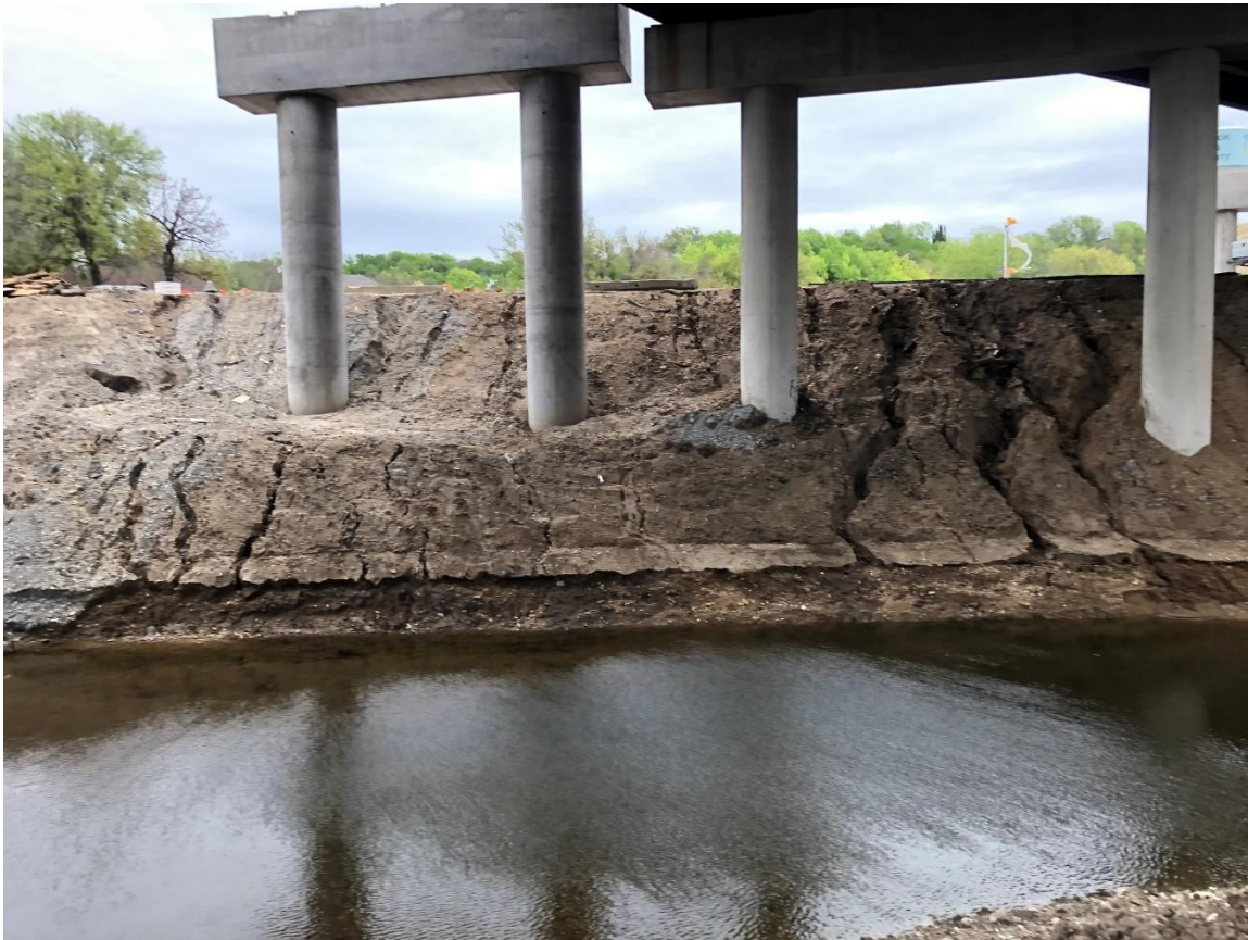
Figure 24- IH-20 project's slope before stabilization.
