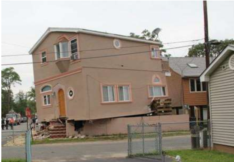
Figure 7: New Foundation Construction Collapses During the Elevation Process (Robbins, 2013)
