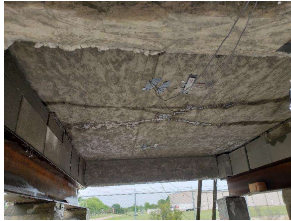
Figure 26: Observed Cracking in Slab
