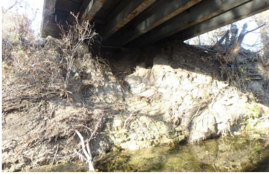
NW channel bank under bridge has moderate erosion and is steep.
