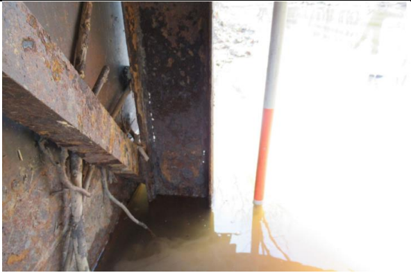
Corroded Web Looking South
