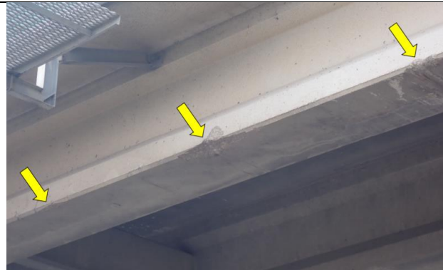
Minor Overheight Impact Spalls of Beam 1 In Span 2, Looking Southwest. (Condition Rating: 6)
