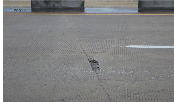
Minor Spall In The Deck Top Surface Along The Bent 4 Joint, Looking Southwest. (Condition Rating: 6)
