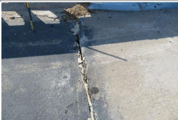
Settlement Right Shoulder Looking South
