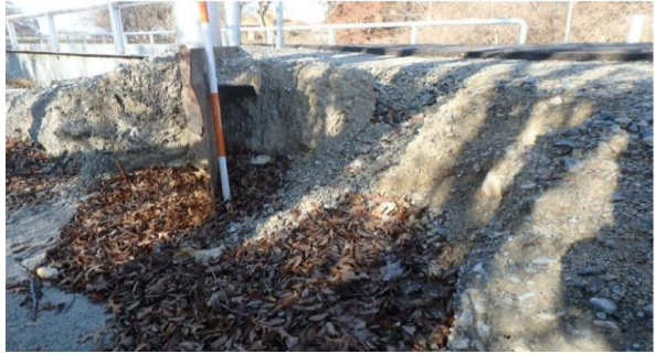
Minor to moderate embankment erosion at south corner of bridge has exposed backside of steel wing wall.
