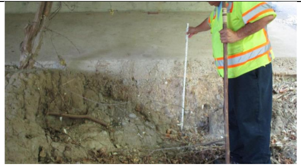
10 - Southeast concrete riprap toe is exposed 30 inches (Looking Southeast)
