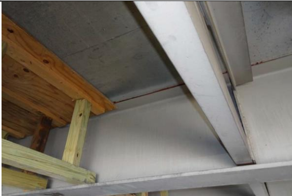
Deck Movement NE Span Looking Southeast
