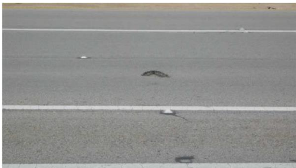
Pothole of 1 sq ft on Deck Pavement
