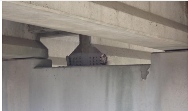
Minor End Delamination/Spalls With Exposed Reinforcement Of Beam 2 in Span 4, Looking Northwest. (Condition Rating: 6)
