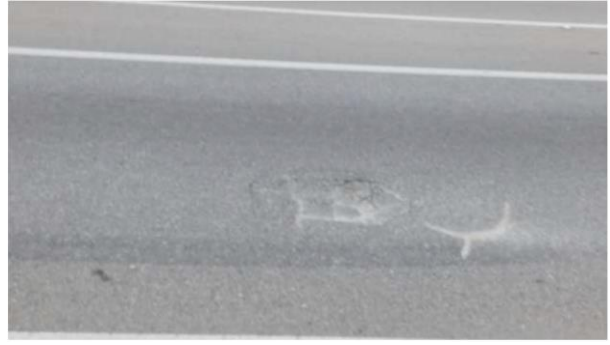
Distressed Area on Asphalt Pavement
