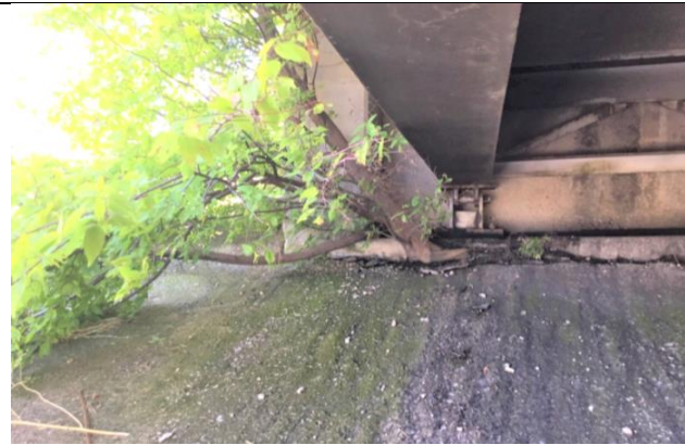
TREE GROWING IN RIP RAP UNDER BRIDGE AT SOUTHEAST CORNER (LOOKING SOUTH)
