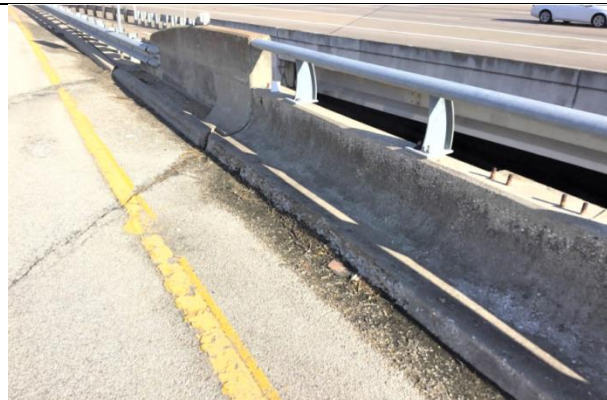
Spalling Along Base Of North Bridge Rail At West Abutment (Looking West)
