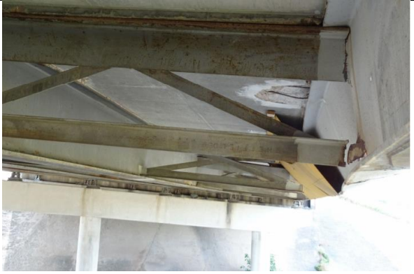
Beam Distortion & Detached Diaphragms Looking South
