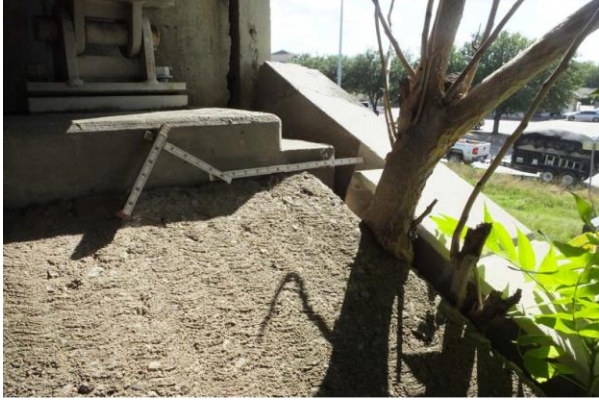
Gap Between SW Riprap and Retaining Wall Looking West
