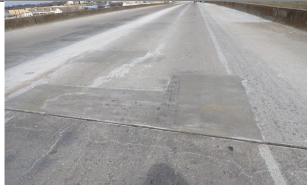
Large Patch in The Span 5 Deck Top Surface at Abutment 6, Looking North. (Condition Rating: 7)
