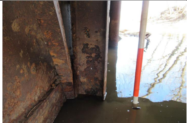
Note: Heavy Rust With Pitting And Flaking On Middle Steel Pile At West Abutment With Small Hole Through Web.
