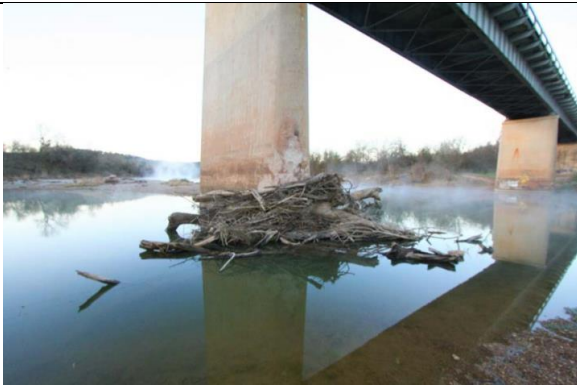
DRIFT AT BENT 5 Looking Southwest
