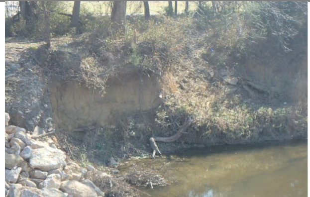
Significant erosion of east upstream bank ~150' from bridge.
