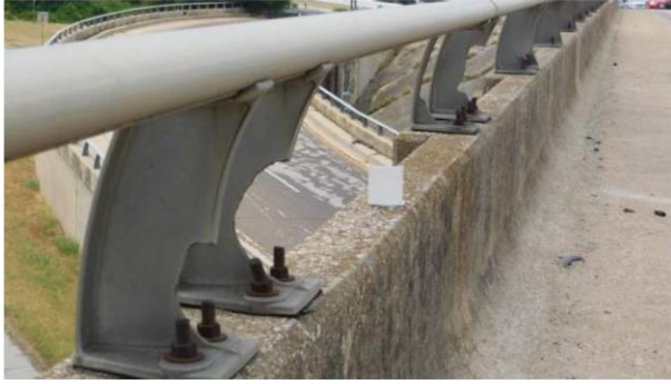
Broken Rail Posts on West Bridge Rail
