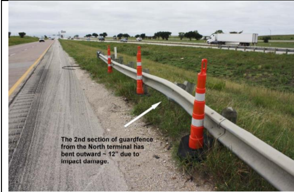
IMPACT DAMAGE N. GUARDFENCE LOOKING NORTH
