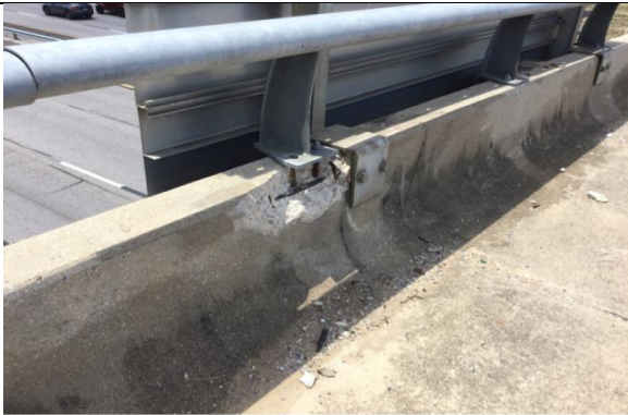
SPALL WITH EXPOSED STEEL IN WEST BRIDGE RAIL OVER BENT 2 FROM SOUTH (LOOKING NORTHWEST)
