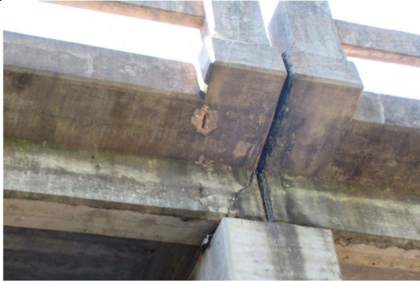
CRACKED T-BEAM Looking Northeast
