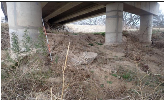
Exposed Column 5 Drilled Shaft At Bent 3 Due To Erosion, Looking North. (Condition Rating: 7)
