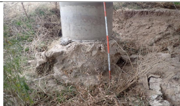
Exposed Column 3 Drilled Shaft At Bent 3 Due To Erosion, Looking Northwest. (Condition Rating: 7)
