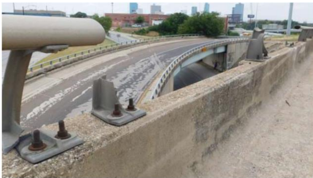
Missing 20 ft tube section on West bridge rail
