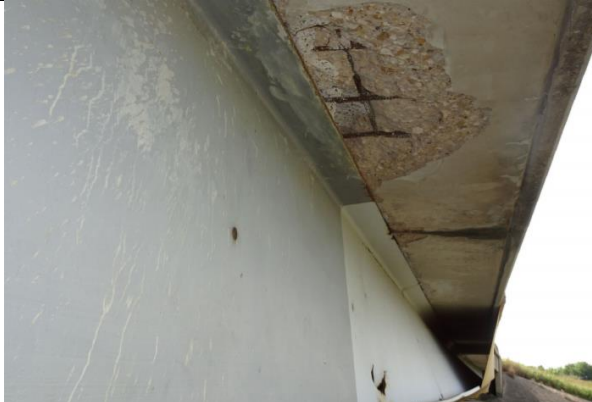
Deck Spall & Hole In Web Looking South
