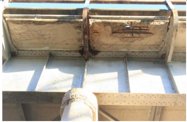
CONCRETE DECK AND CAP DETERIORATION Looking North
