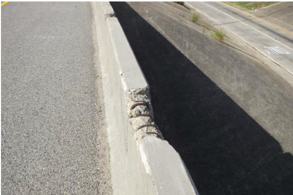
Spalled SE Bridge Rail Span 1 From SW Looking Northeast
