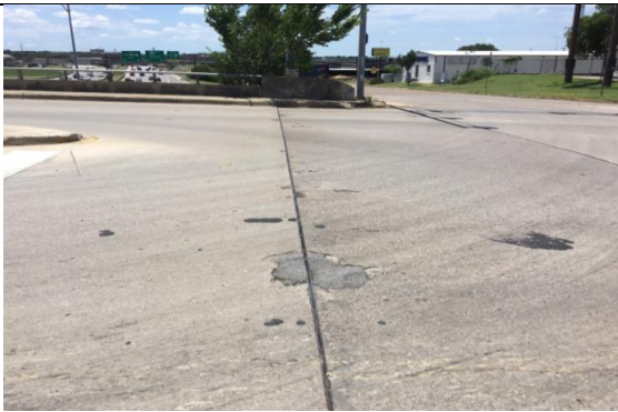
SPALLING ALONG NORTH ABUTMENT JOINT (LOOKING WEST)
