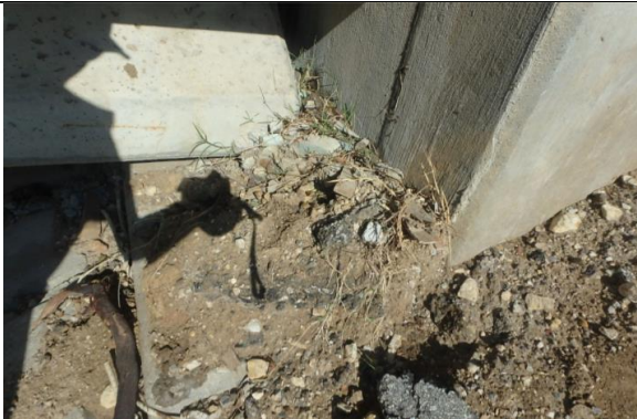
Dirt and construction debris around girder bearing at east abutment.
