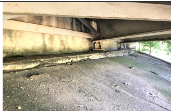
Settlement Of Rip Rap At East Abutment Cap (Looking South)
