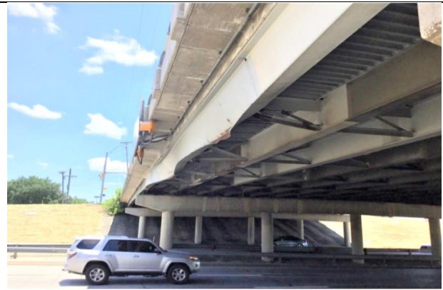
IMPACT DAMAGE TO EAST EXTERIOR BEAM IN SPAN 3 FROM SOUTH OVER SH 121 SB LANES (LOOKING SOUTH)
