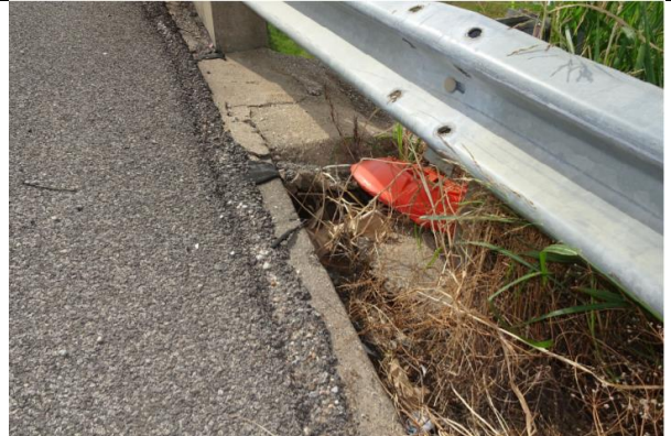
Erosion At Nw Corner Embankment Looking Southwest
