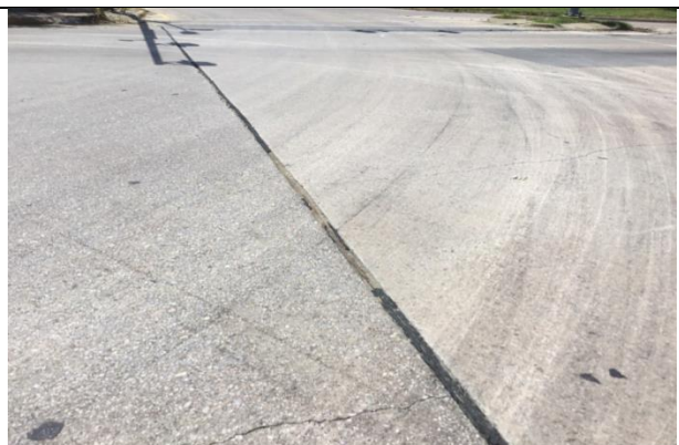
DETERIORATION OF NORTH RELIEF JOINT (LOOKING WEST)
