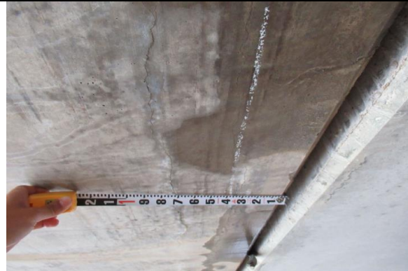
CRACKED BEAM Looking West
