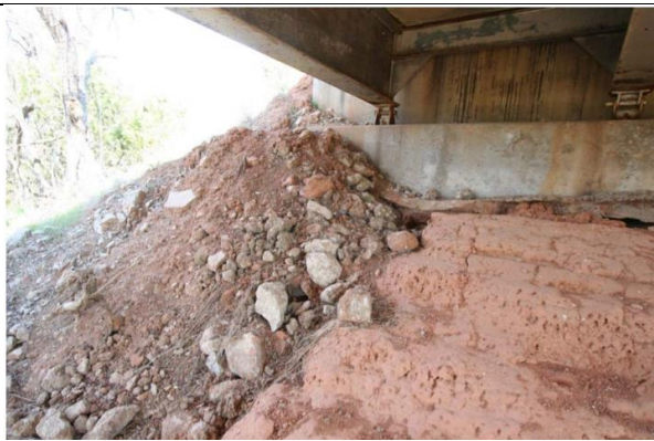
EROSION REPAIR AT NORTH ABUTMENT Looking Northwest
