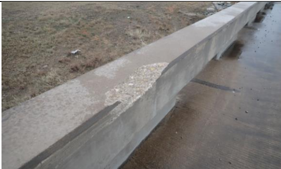
24" Long By 8" Wide By 1" Deep Spall In The Northeast Bridge Railing In Span 4, Looking East. (Condition Rating: 7)
