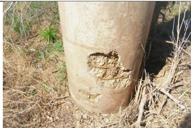
SPALL AT EAST COLUMN BENT 4 Looking North
