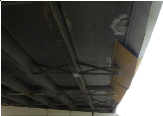
Overheight Impact Span 2 (Center) Looking South
