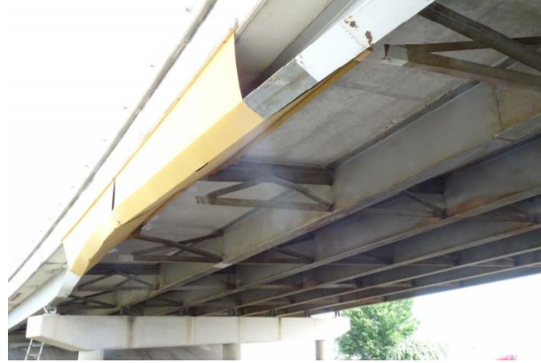
Overall Impact W. Exterior Beam W/ Tarp Looking Northeast
