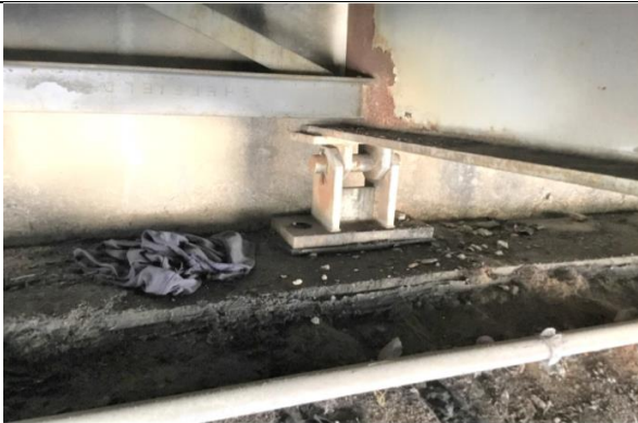
MISSING ANCHOR BOLT AND NUT AT BEARING 11 FROM WEST AT NORTH ABUTMENT (LOOKING NORTH)
