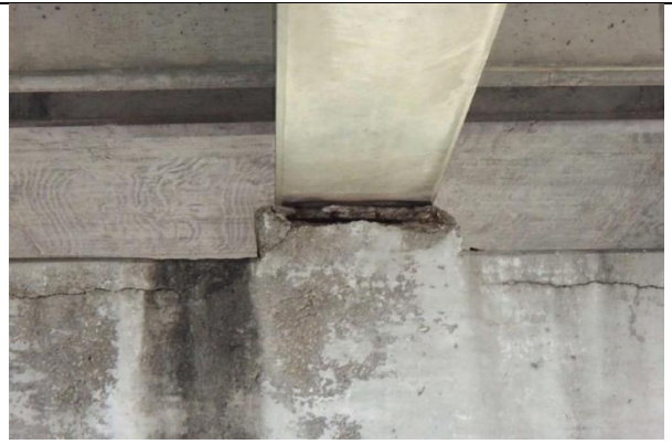
BEARING PEDESTAL SPALLS Looking South
