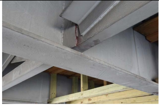
Cracked Diaphragm Weld NE End Span Looking North
