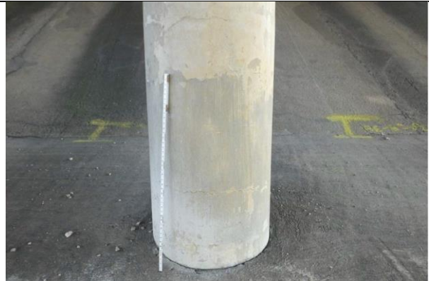
Horizontal Column Crack Bent 2 From SW Looking Southwest
