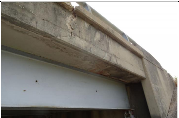
Impact Crack & Spall E Railing At N End Looking Northwest
