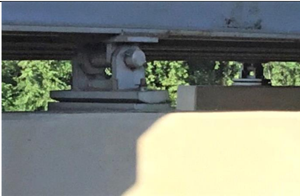
Missing Nut For Anchor Bolt On North Bearing At Bent 7 From West (Looking Southwest)
