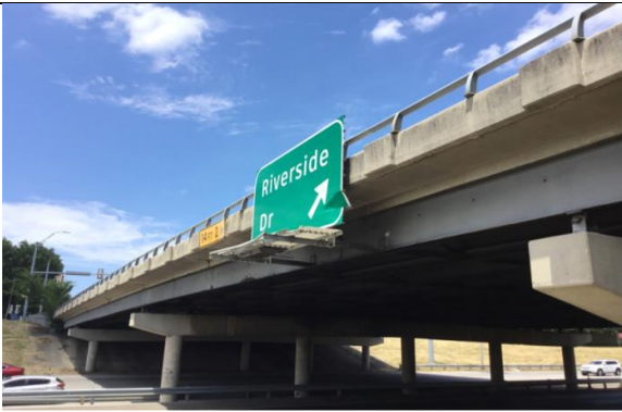
IMPACT DAMAGE TO STREET SIGN ATTACHED TO WEST BRIDGE RAIL OVER SH 121 NB LANES (LOOKING NORTH)
