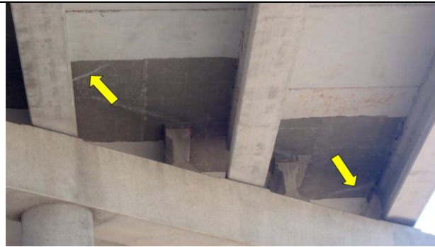
Minor diagonal cracks with light efflorescence in the deck soffit at Bent 6, looking east. (Condition Rating: 8)
