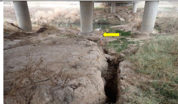
Moderate Erosion Gullies In The Southeast Overbank In Span 3, Looking Northwest. (Condition Rating: 7)
