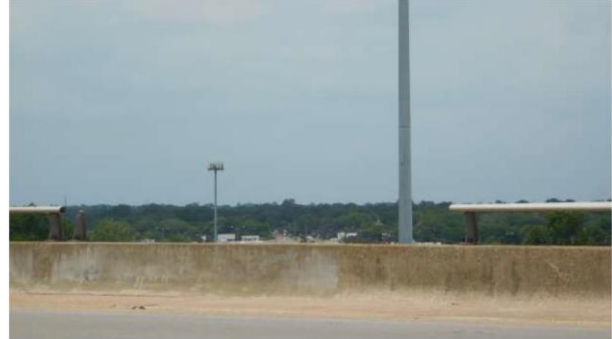
Missing 20ft Tube Section on East Rail Bridge
