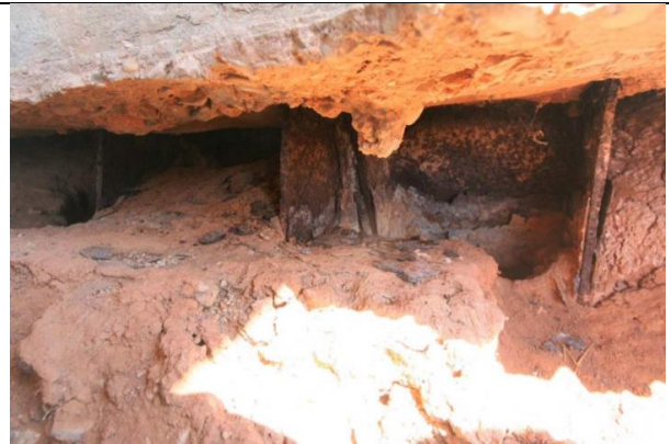
RUSTED STEEL PILING AT NORTH ABUTMENT Looking North
