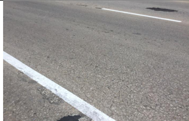
MAP CRACKING ON ASPHALT SURFACE IN SOUTH SPAN (LOOKING SOUTHWEST)
