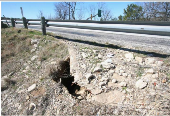
EROSION HOLE AT NE SHOULDER Looking Southwest
