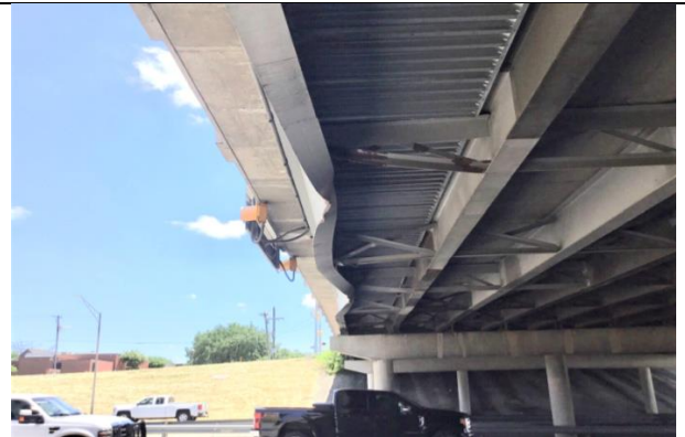
CLOSE UP OF DAMAGE TO EAST EXTERIOR BEAM IN SPAN 3 FROM SOUTH OVER SH 121 SB LANES (LOOKING SOUTHEAST)
