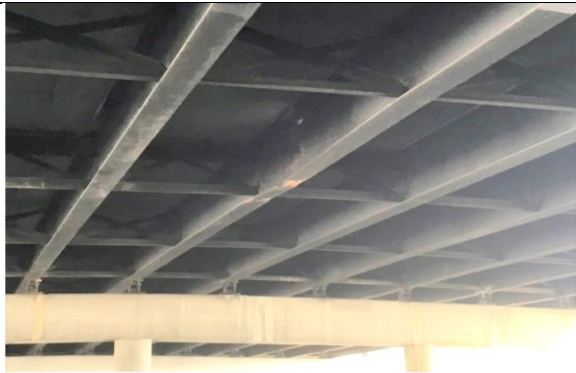
DAMAGED BEAM 8 FROM EAST AT SPAN 3 FROM SOUTH (LOOKING SOUTH)
