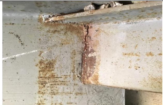
South Diaphragm Has A Cracked Connection To Web Of Beam 4 From North Over East Abutment (Looking North)
