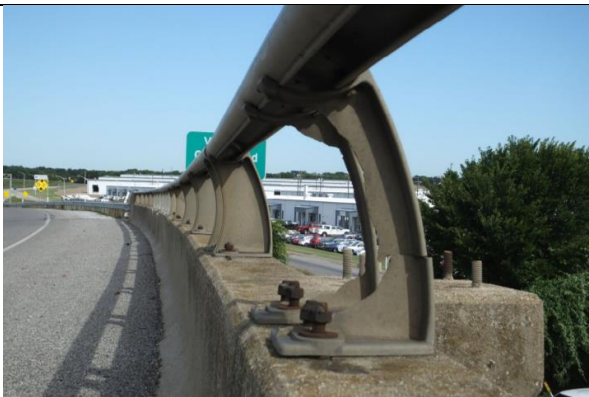
Tube Rail Damage Looking North
