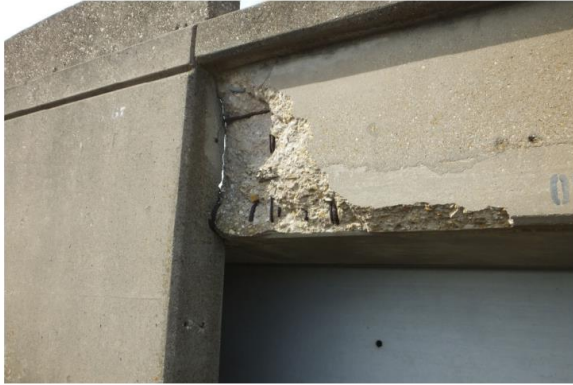
Spall @ Se Bridge Corner Looking Southwest
