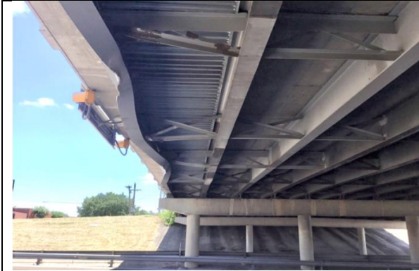
TWISTING OF BEAM 2 FROM EAST IN SPAN 3 FROM SOUTH (LOOKING SOUTH)
