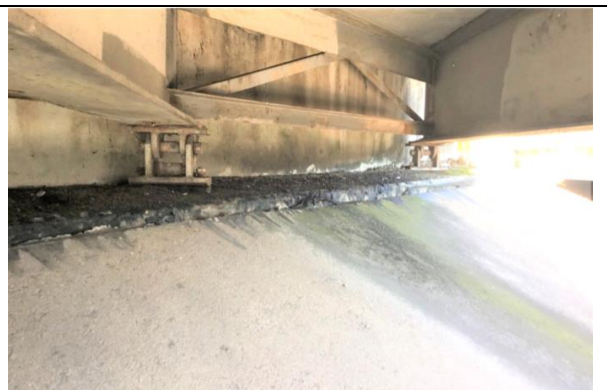
Settlement Of Rip Rap At West Abutment Cap (Looking North)
