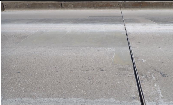
Large Patch in The Span 4 Deck Top Surface at Bent 4, Looking West.
