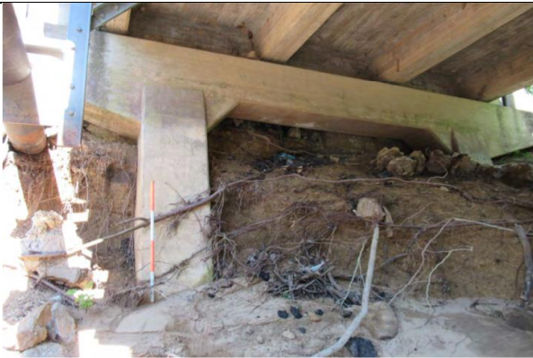
EROSION Looking Southeast
