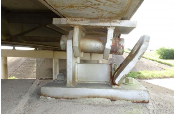
Damaged W. Bearing Bent 2 From North Looking South
