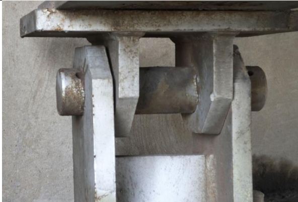
Missing Cotter Pins Nw Abutment Looking North
