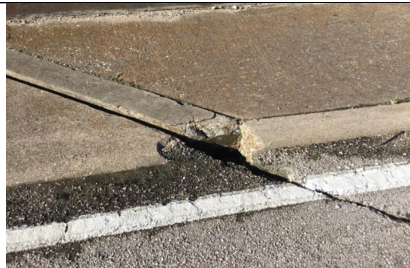
Spall In West Approach Slab At Southeast Corner (Looking Southwest)
