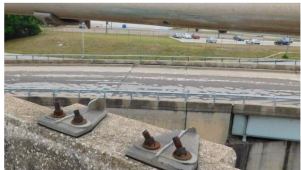
Missing posts on West bridge rail
