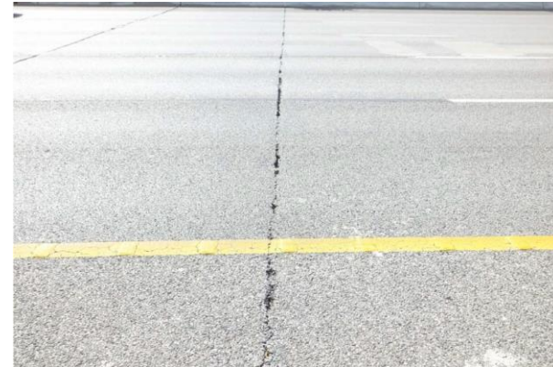
Minor Deterioration Along SW Abutment Joint Looking Northwest
