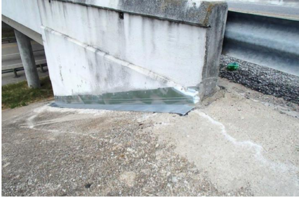
EROSION REPAIR Looking Northeast
