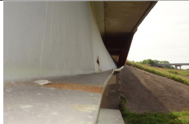
Gen. Beam Distortion & Tarp Looking South
