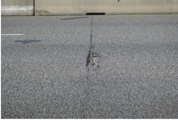
Pothole In Deck Span 2 Looking West
