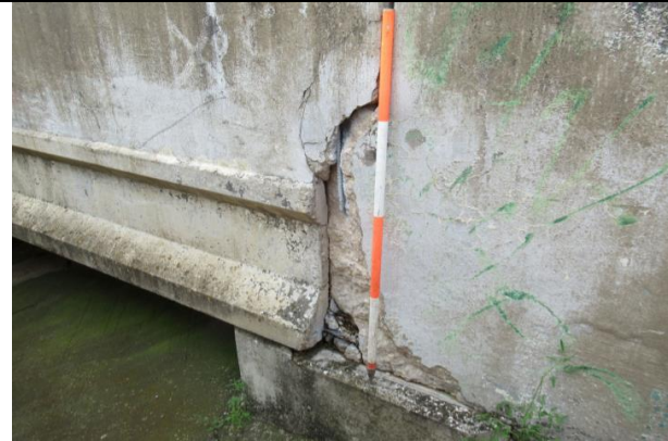
SPALLED WINGWALL Looking Southeast
