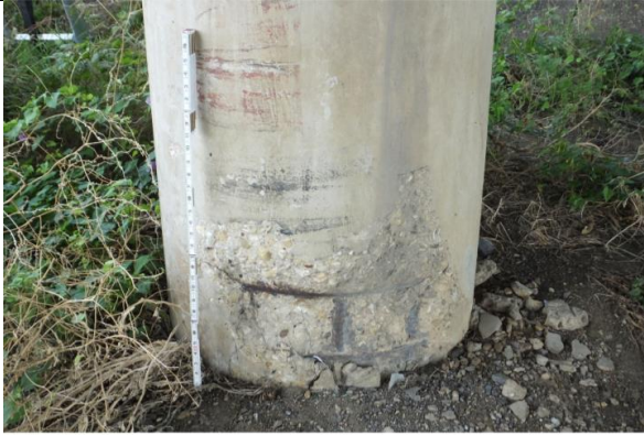
W. Exterior Column Base Spall Looking North
