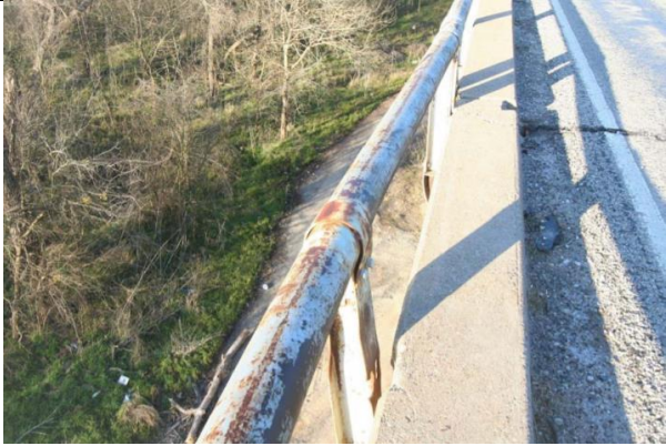
DAMAGED RAIL Looking West
