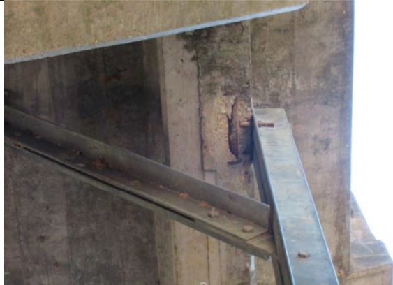
SPALLED T-BEAM Looking West
