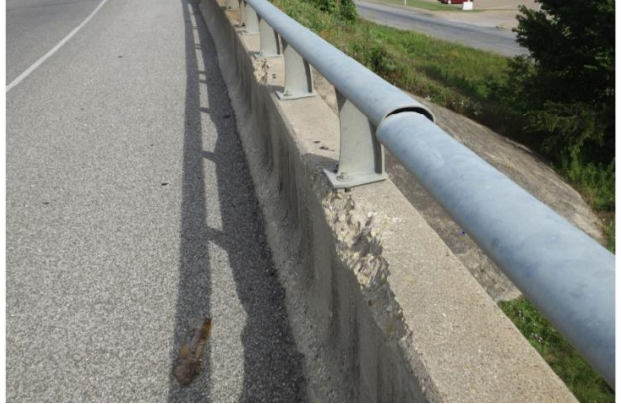
East Concrete Bridge Rail Spall Looking North
