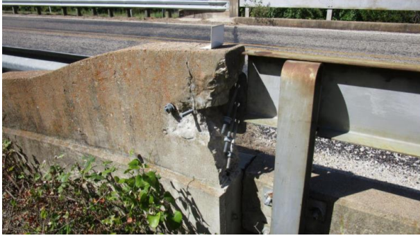
9 - East corner wingwall is spalled at rail connection, 3 bolts completely loose (Looking Southwest)
