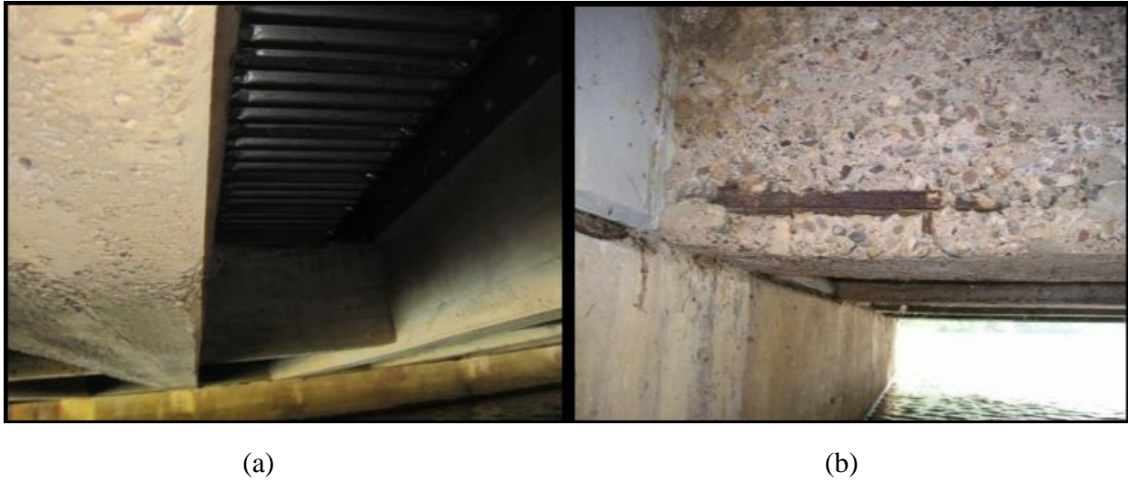
Figure 4-3: Typical Concrete Encasement Condition (Left), Localized Spalling of Concrete Encasement (Right) (NJDOT, 2015)
