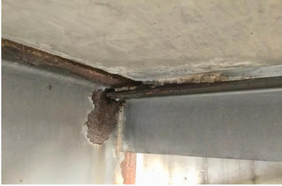
PACK RUST BETWEEN BEAM END DIAPHRAGM AT SOUTH ABUTMENT (LOOKING SOUTHEAST)
