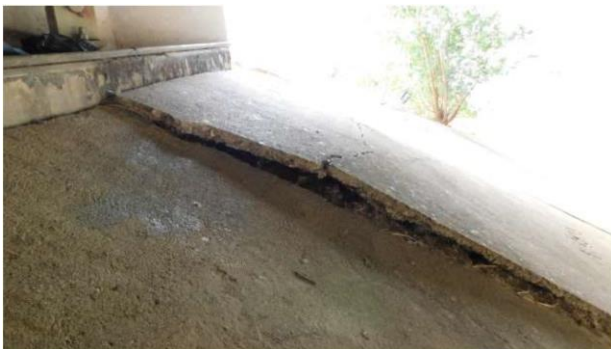
Northeast riprap heaving
