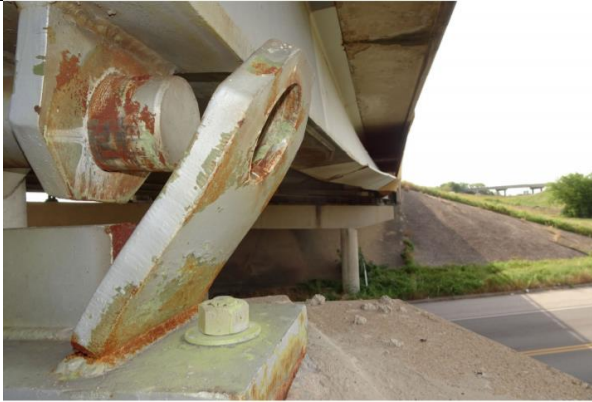
Damaged West Bearing & Beam Looking South
