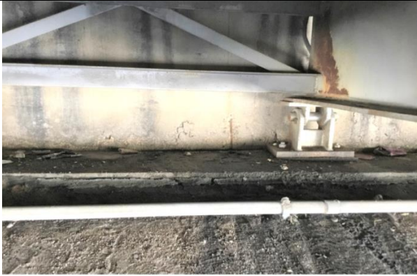
SPALLING WITH EXPOSED STEEL IN NORTH BACKWALL NEAR BEARING 12 FROM WEST (LOOKING NORTHWEST)
