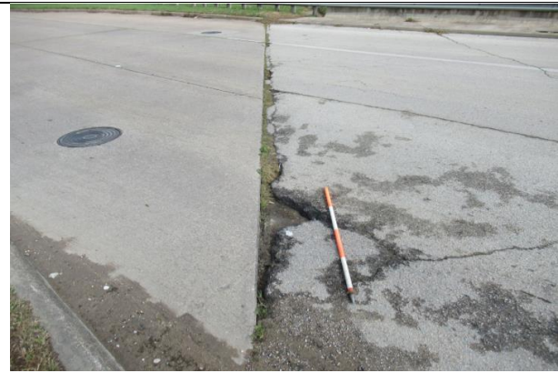
SPALLED ASPHALT Looking Northwest
