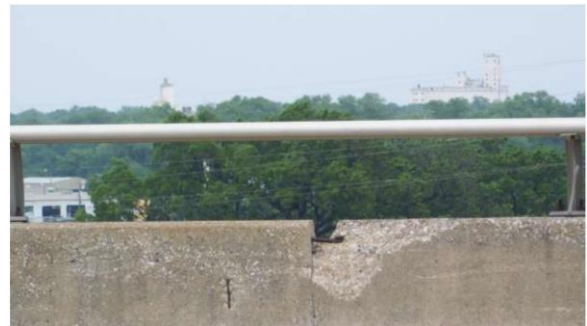
Spall on East Parapet
