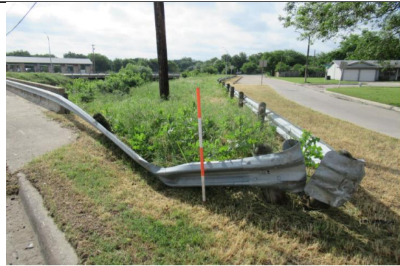
DAMAGED GUARDFENCE Looking Southeast
