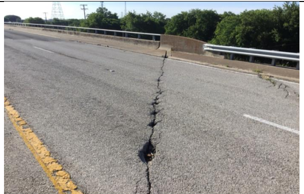
Asphalt Spalling Above West Abutment Joint (Looking Southeast)
