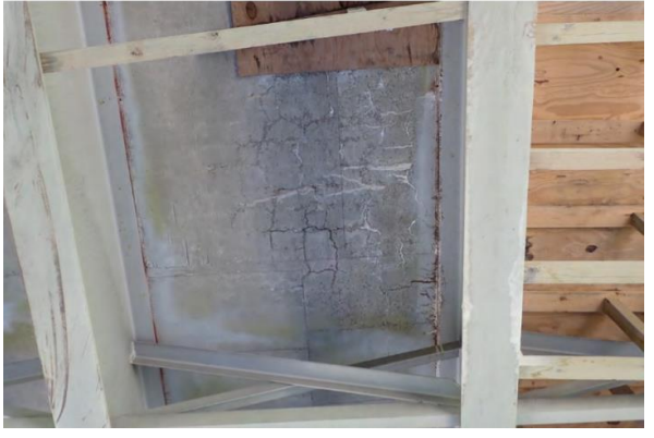
MODERATE MAPPING CRACKS IN BOTTOM OF DECK Looking North
