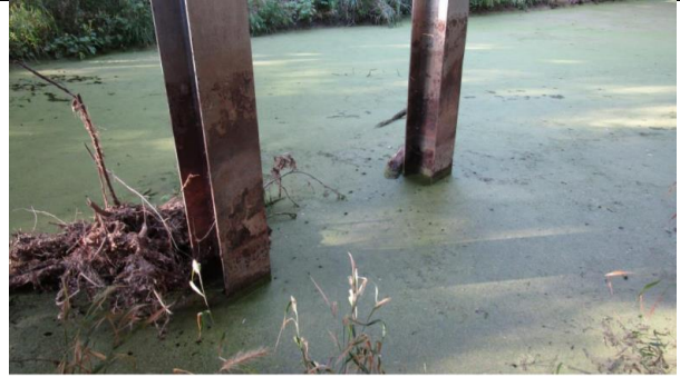
8 - Piles at bent 2 have rusting and flaking near water line (Looking South)
