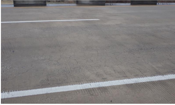
Hairline Map Cracks With Caving In The Deck Top Surface In Span 3, Looking Southwest. (Condition Rating: 6)
