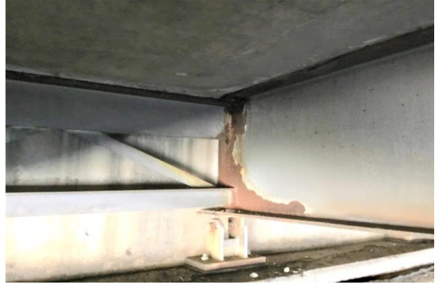
RUSTING OF STEEL MEMBERS AT SOUTH ABUTMENT (LOOKING SOUTHWEST)
