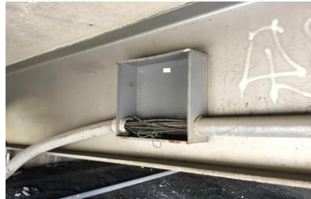
MISSING ELECTRICAL BOX COVER ON BEAM 2 FROM WEST AT NORTH ABUTMENT (LOOKING EAST)
