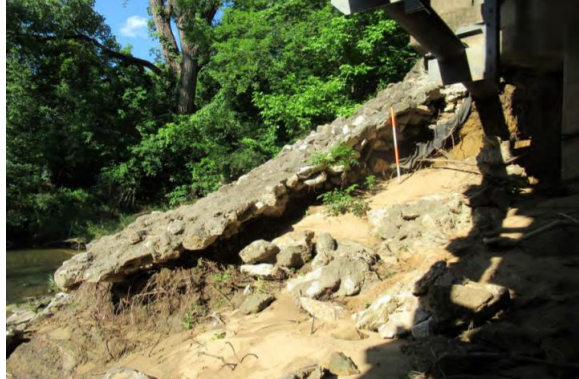
UNDERMINED RIPRAP Looking Northeast
