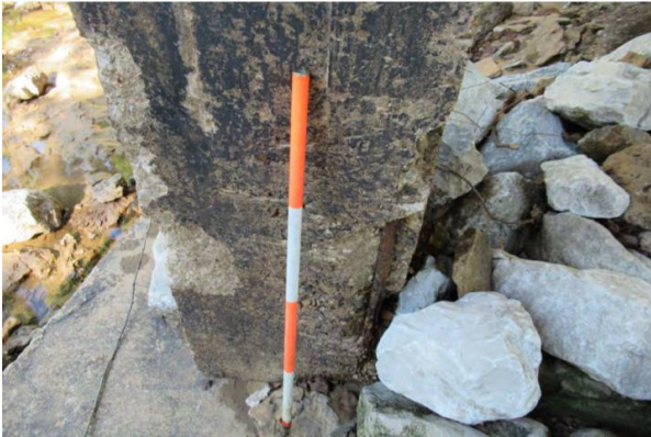
SPALLED COLUMN Looking East
