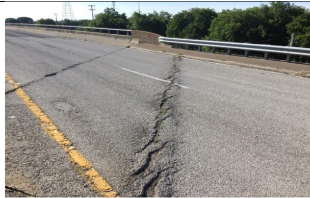
Asphalt Cracking At West Relief Joint (Looking Southeast)
