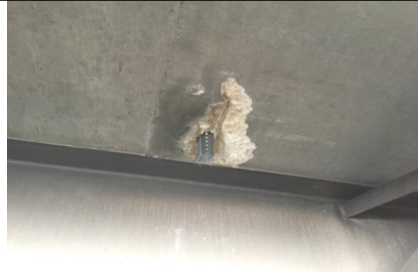
SPALL WITH EXPOSED STEEL IN DECK SOFFIT AT SOUTH SPAN (LOOKING SOUTHEAST)
