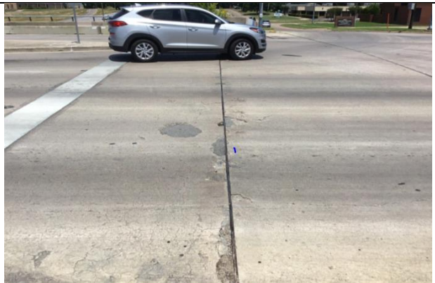
SPALLING ALONG SOUTH ABUTMENT JOINT (LOOKING EAST)
