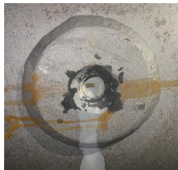
Figure 3.22 1-inch Hole Spanning Pipe Sample
