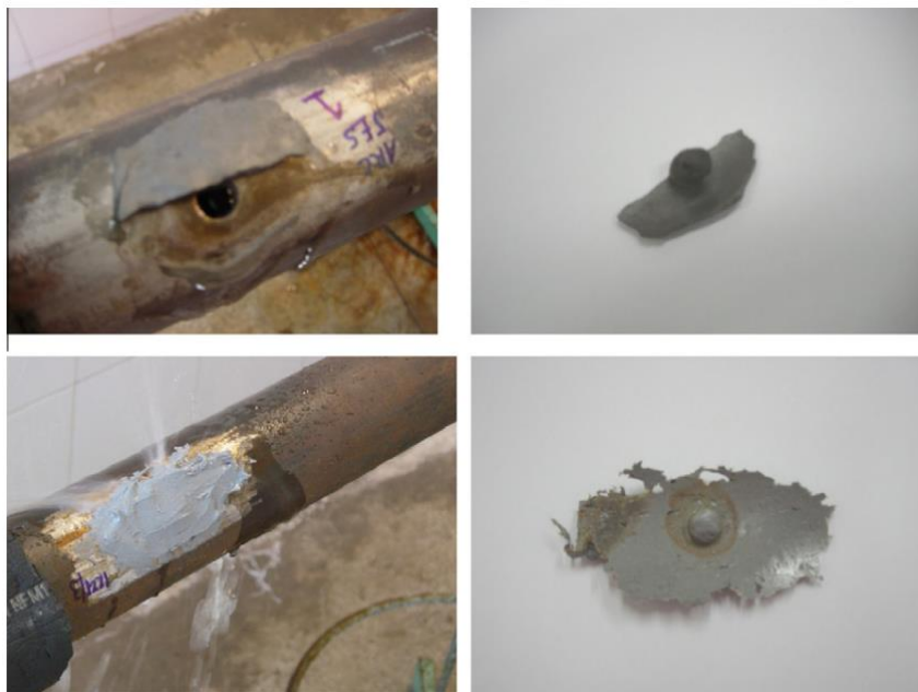
Figure 2.5 Corrosion Damaged Pipes Repaired with Epoxy (Costa Mattos et al., 2012)
