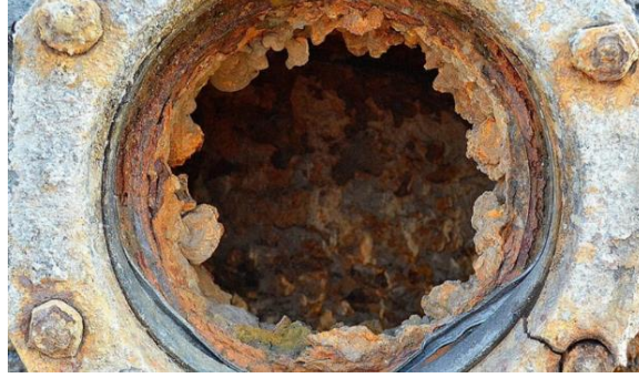
Figure 1.5. Pipe with Corrosion Deposit Affected Hydraulic Flow Capacity (Source: APP Manufacturing)
