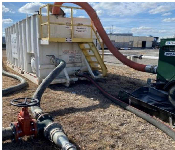
Figure 4.11 Test Setup End Loop Connection to Water Tank
