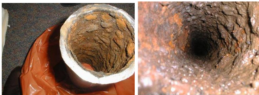
Figure 5.40 Nuclear Service Water System Piping Tubercles Increased Pipe Roughness and Reduce Pipe Internal Diameter (Adapted from Onat et al., (2016))
