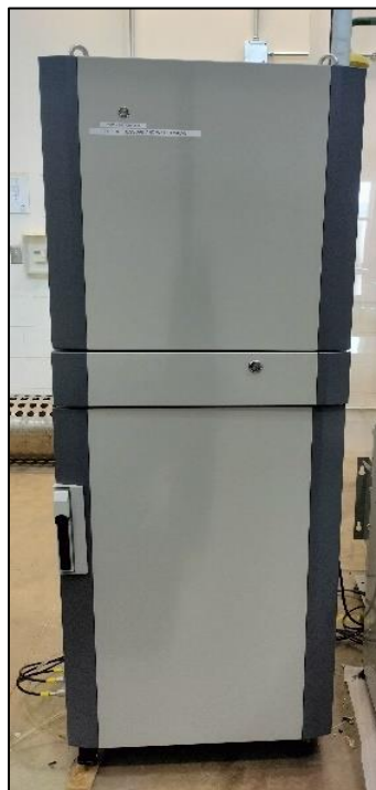
Figure 3.37 Control Panel Unit
