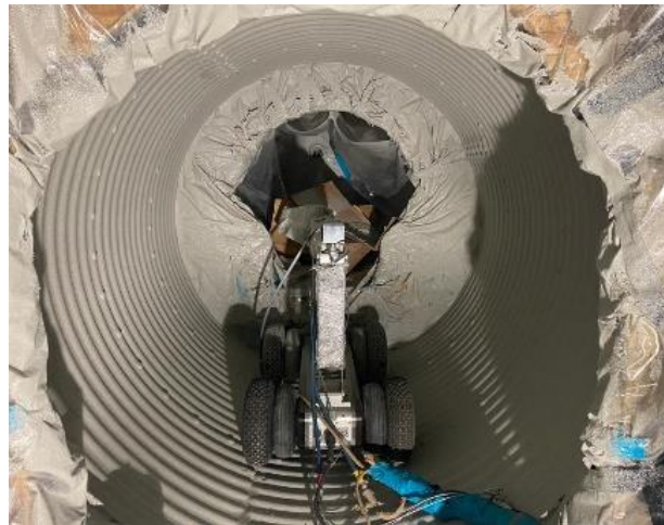
Figure 1.10 SAPL Robotic Application
