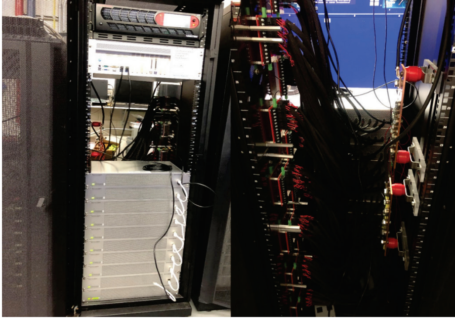
Figure 42. Front and back of one of the BMS testbed cabinets
