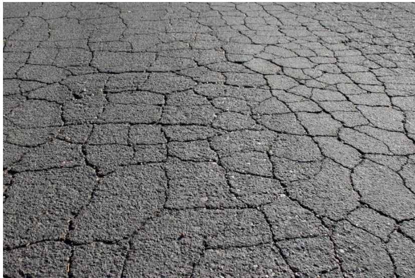
Figure 2.28 Fatigue cracking of asphalt pavement
