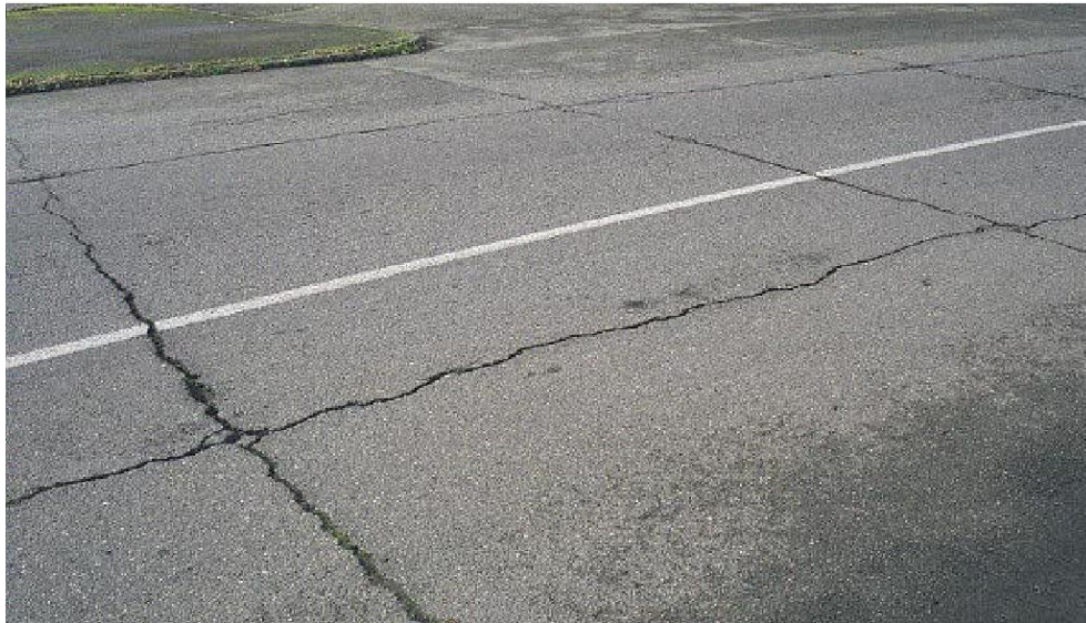
Figure 2.29 Low Temperature Cracking (Ahmad and Khawaja, 2018)
