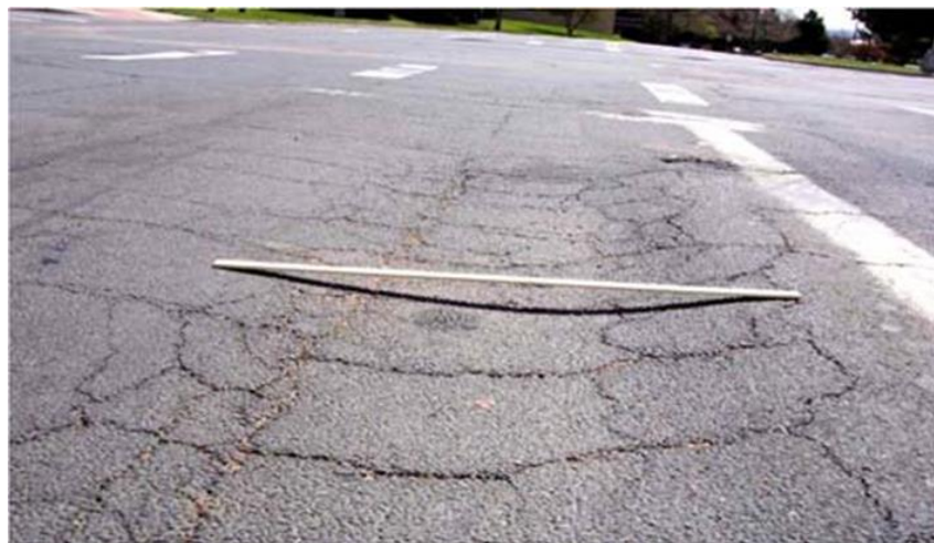
Figure 2.27 Rutting of pavement (Sarah et al 2017)
