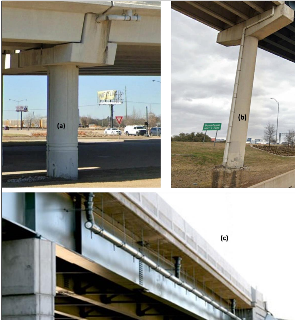
Figure 2.4. Closed bridge deck drain (a) Drain embedded within bridge structure (GoogleEarth, 2022) (b) Drain running down the exterior of the bridge (GoogleEarth, 2022) (c) Combined drains which discharge at bridge ends (Hennegan and Associates, 2020)
