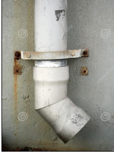
Figure 2.7. Rust stains may indicate fracture or a loose joint (Dreamstime, 2022)
