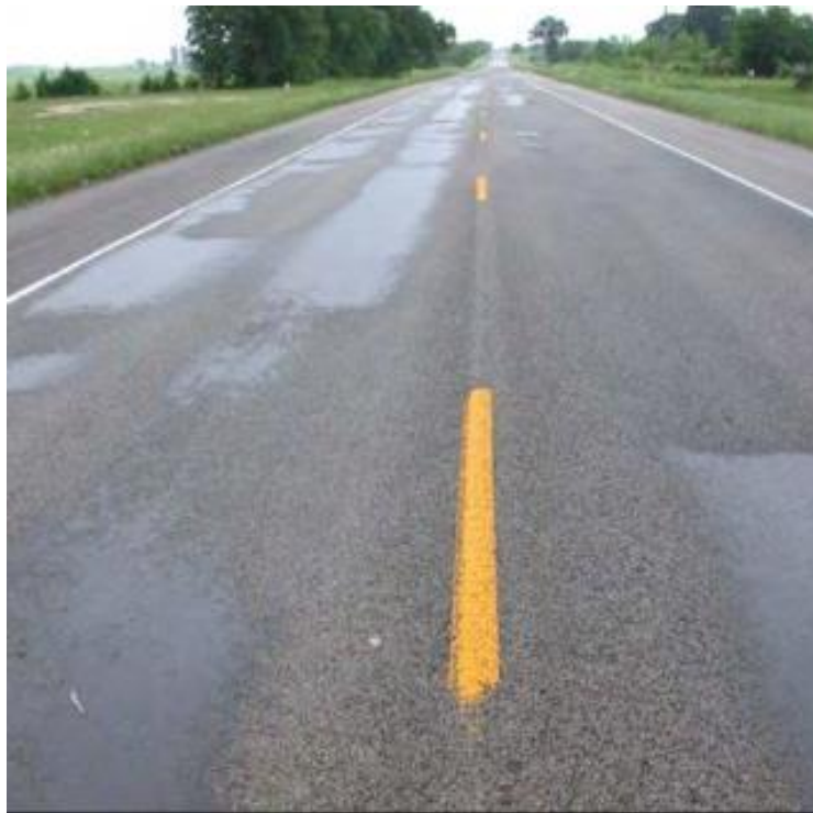
Figure 2.12. Bleeding on pavement (Lawson et al, 2007)
