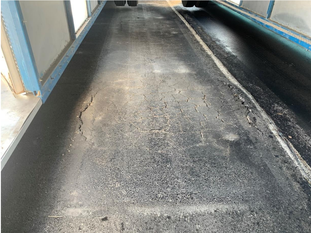
Figure 3.80 Surface cracking on section O after 350,000 passes
