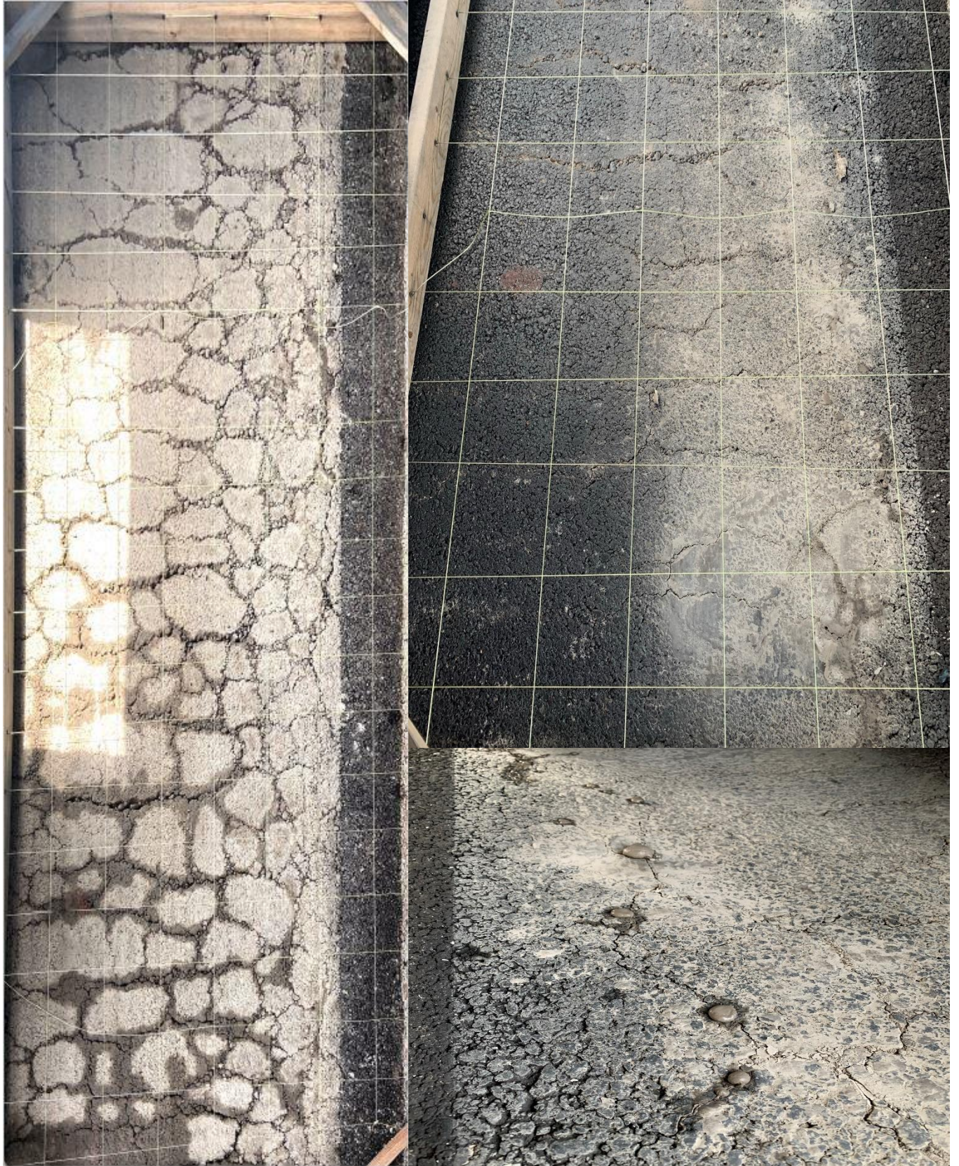
Figure 3.82 Surface cracking on section T (left) and S (right) after 57,000 passes
