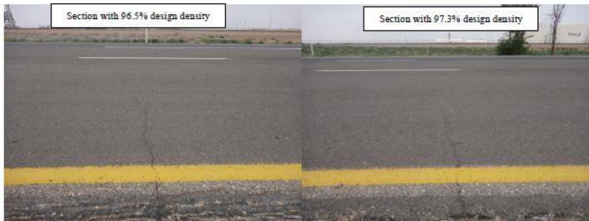
Figure 2.21 Reflective cracking of RAS test sections on US87, Amarillo (Zhou et al. (2013).
