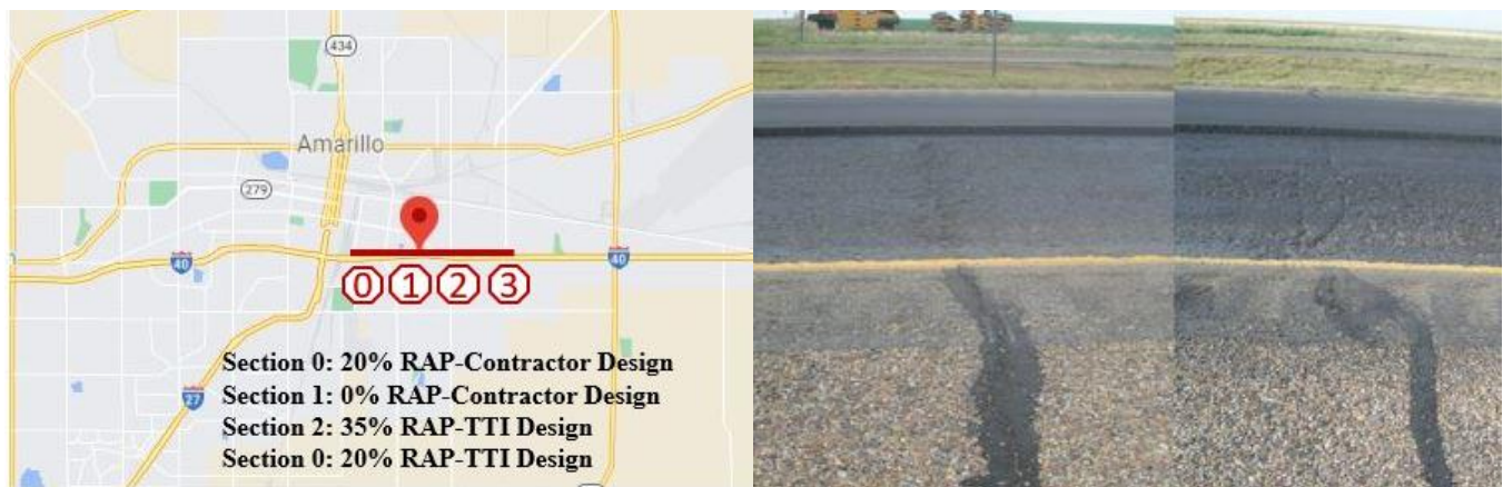
Figure 2.19 I-40 Experimental sections. Location and existing pavement condition after 4” milling, Zhou et al., (2011)
