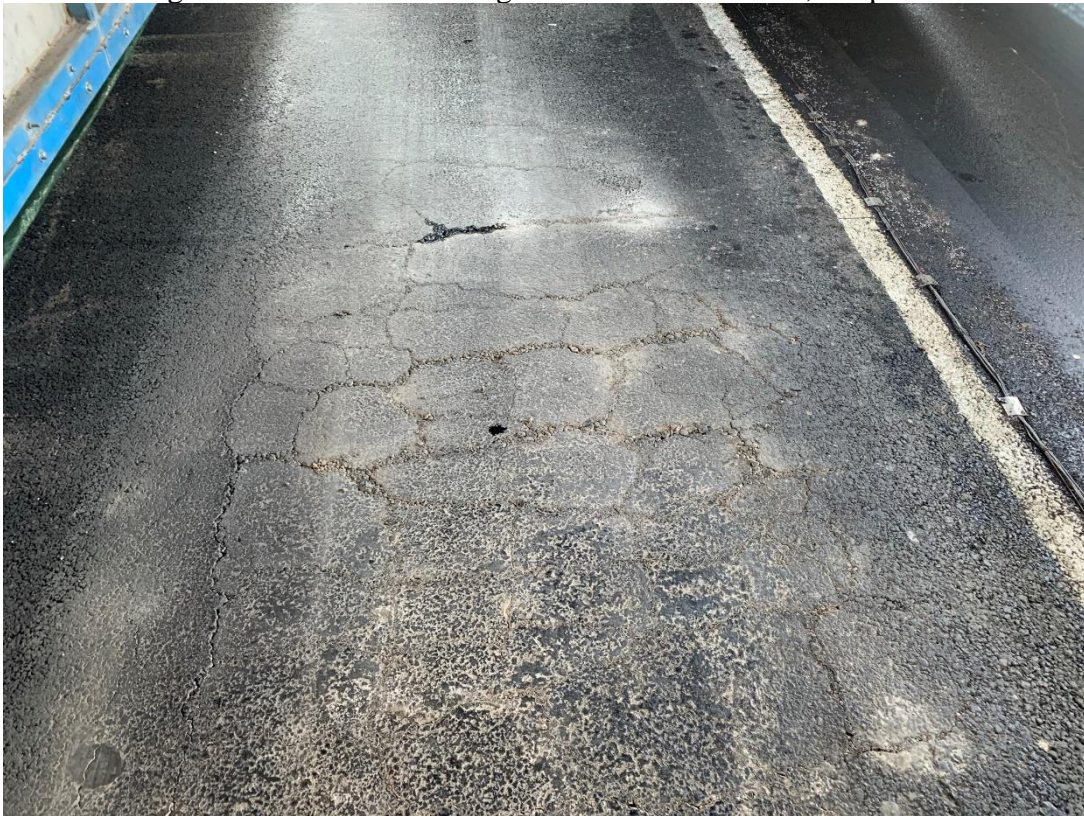
Figure 3.81 Surface cracking on section P after 350,000 passes
