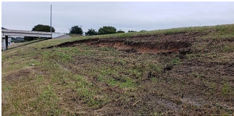
Figure 3.3 The failed section at I-20 and Parks Springs Blvd
