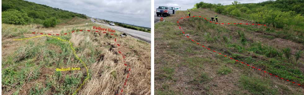
Figure 3.2 The failed sections at US-287 (after Islam 2021)
