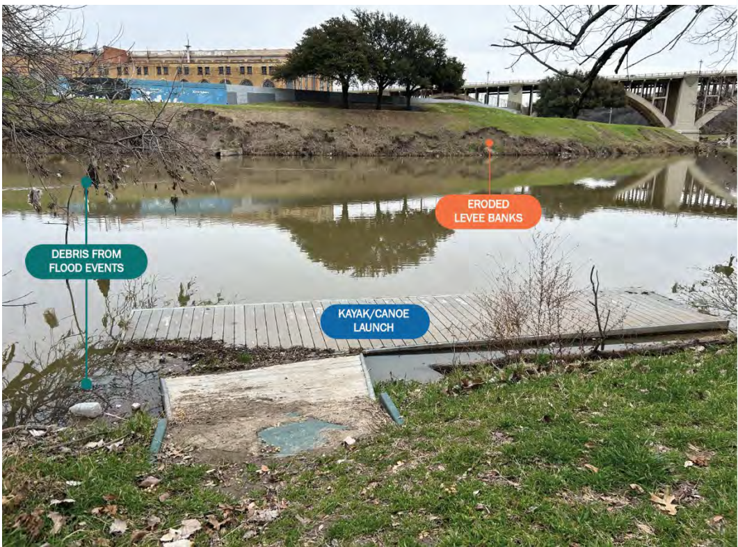
Figure 40 Flood Damaged Dock (Adapted with Illustrator)
