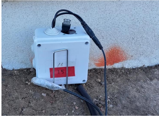
Figure 10: Natural Gas detectors placed at the Urban testbed next to the Structure foundation. The sensor was placed on the soil surface to orient faces with wire meshes along vertical axis. Top surface is having a port for computer connection and power supply wire while bottom is a levelled surface.
