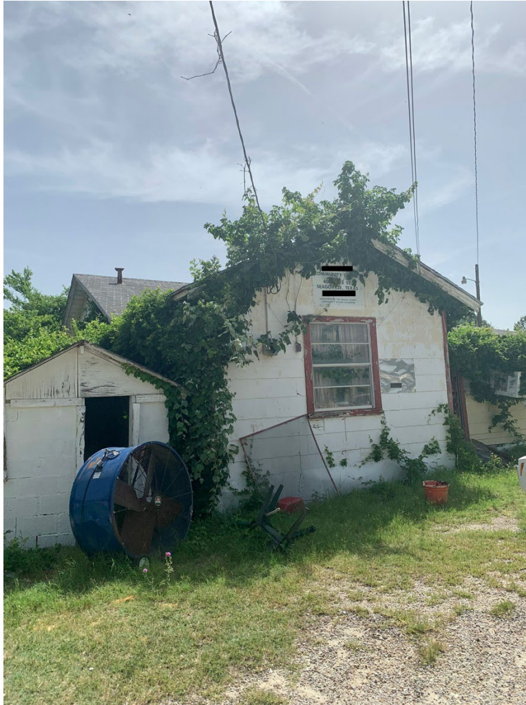
Figure 4.5: The old community center that used to host community gathering events. It currently sits abandoned on the inside due to its poor building conditions but hosts bar-b-que events and other social gatherings on the outside. Note: Perez Vela, J. (n.d.)
