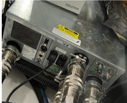
Figure 2.2: Coolant Distribution Unit
