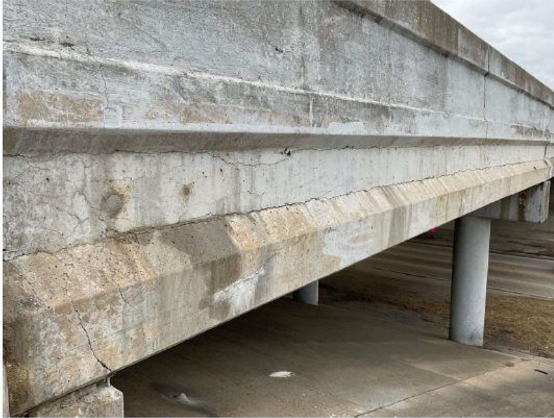
PHOTO 2 Recommended Maintenance Needs
